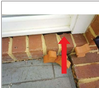
The void below the master bedroom sliding glass door needs to be sealed by a qualified contractor.
