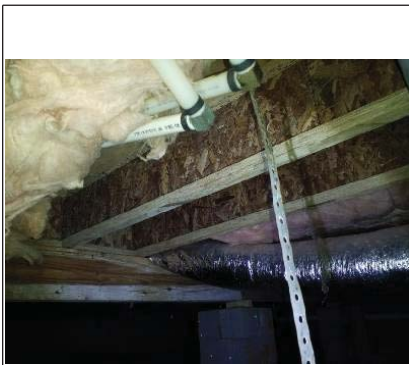
The missing basement crawlspace insulation need to be replaced by a qualified contractor.
