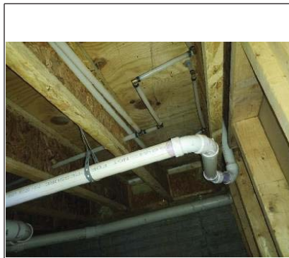
The missing garage crawlspace insulation needs to be installed by a qualified contractor.
