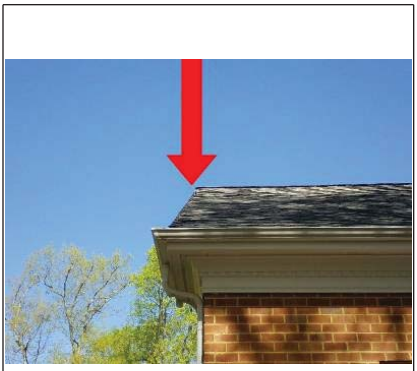
The nail pops on the garage need to be repaired by a qualified contractor.
