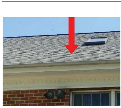
Recommend having a qualified contractor repair the nail pop on the back roof section.
