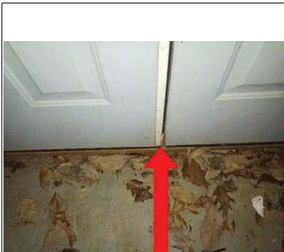
The basement door needs new weather stripping installed.
