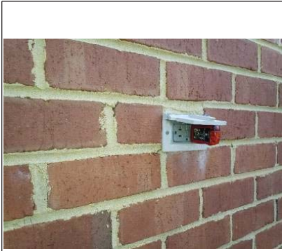
The GFCI receptacle above the patio needs to be wired correctly by a licensed electrician.
