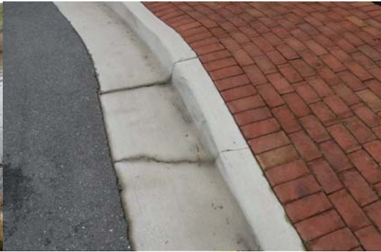
Curb Section with Crack
